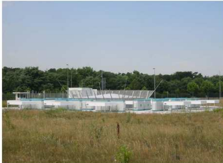
Figure 2-5: The Wind Temperature Radar (WTR) as installed at Frankfurt Airport intended to be used for the WSWS. The system provides wind velocity and temperature up till 1500 m height by combining Doppler-Radar for clear air measurements and Radio Acoustic Sound System (RASS) for measurements in bad weather
